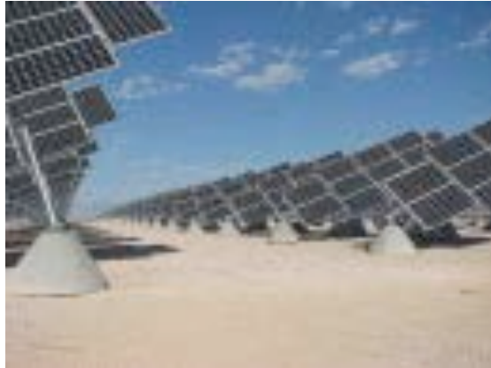
Figure A-6. 15 MW Large-Scale Photovoltaic Power Plant, Nellis Air Force Base, Nevada (Photo: Courtesy of Sunpower Corp.)
